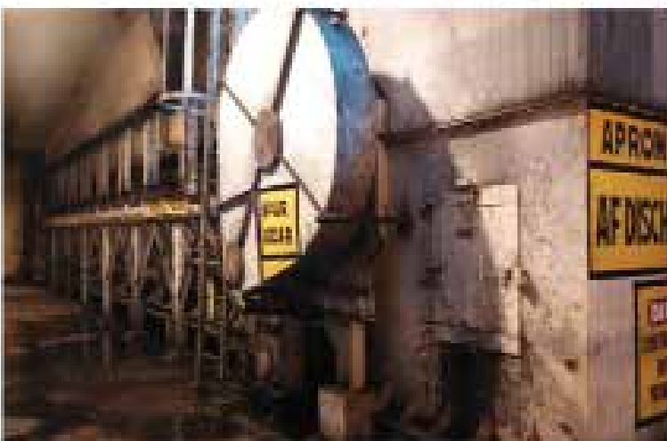
Apron Feeder - Bottom of Wagon Tippler Complex
